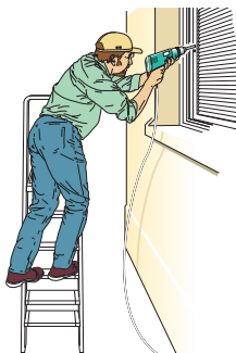
Figure 2a Incorrect - steps side-on to work activity
